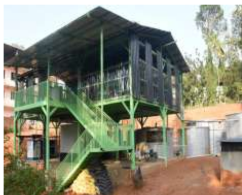
1 MLD STP at Kozhikode medical College
