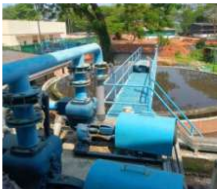
500 KLD STP at Kozhikode medical College
